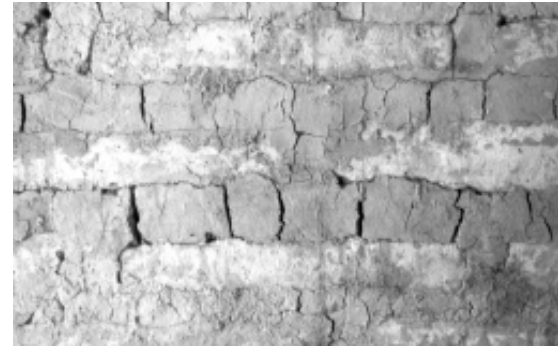
Bad workmanship – thick layers of plaster in this case – are often the real cause of failure in an earthquake.
