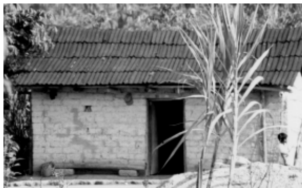
Asphalt impregnated sheets tend to warp and de-laminate in tropical conditions
