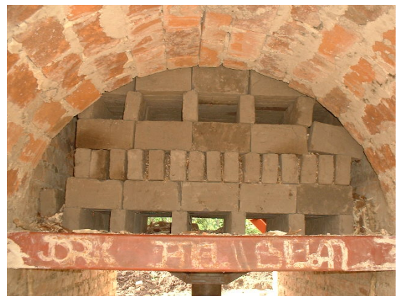
Vertical shaft brick kiln in Nicaragua
